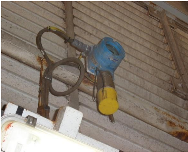
Figure 1 H 2 S gas detector was mounted at height.
