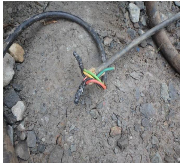
Figure 2: Cable terminations / entries with sheathing cut short, and splices with only electrical tape, including cable repairs using electrical tape.
